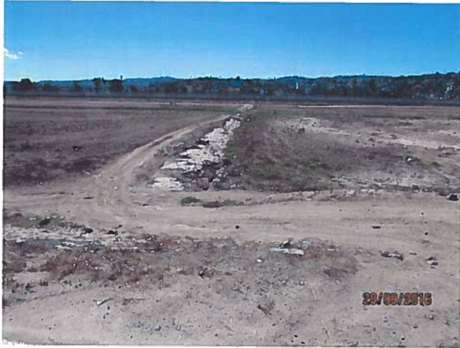
Energy dissipator between the North and South Levees. Access road comes off of the North Levee for the border patrol to use.
