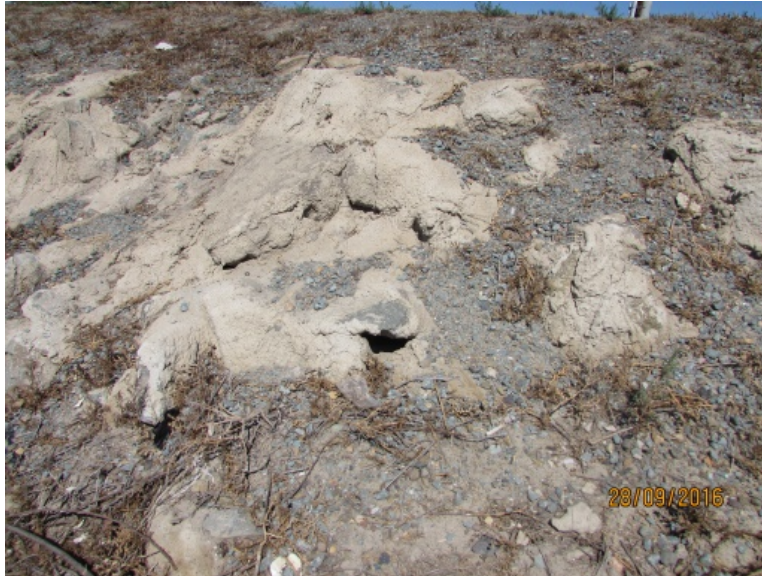
Ground squirrel burrows along the north levee.
