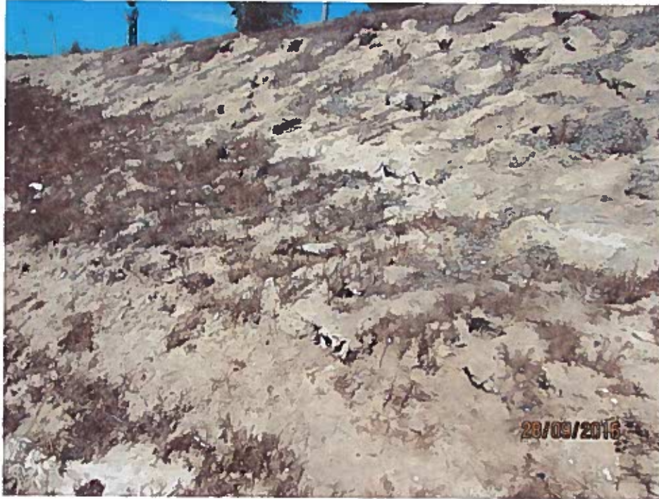
Ground squirrel burrows along the North Levee.
