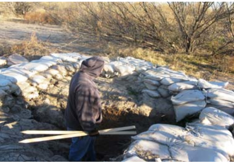
Large sand boil near Station 7+000 on landside of levee (picture courtesy George Sills).
