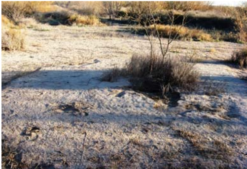
Sand boil near Station 7+000 on landside of levee (picture courtesy George Sills).
