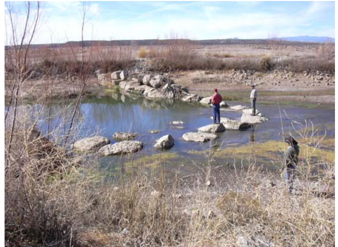
Photo 11. View of existing vortex weir showing scoured area downstream.
