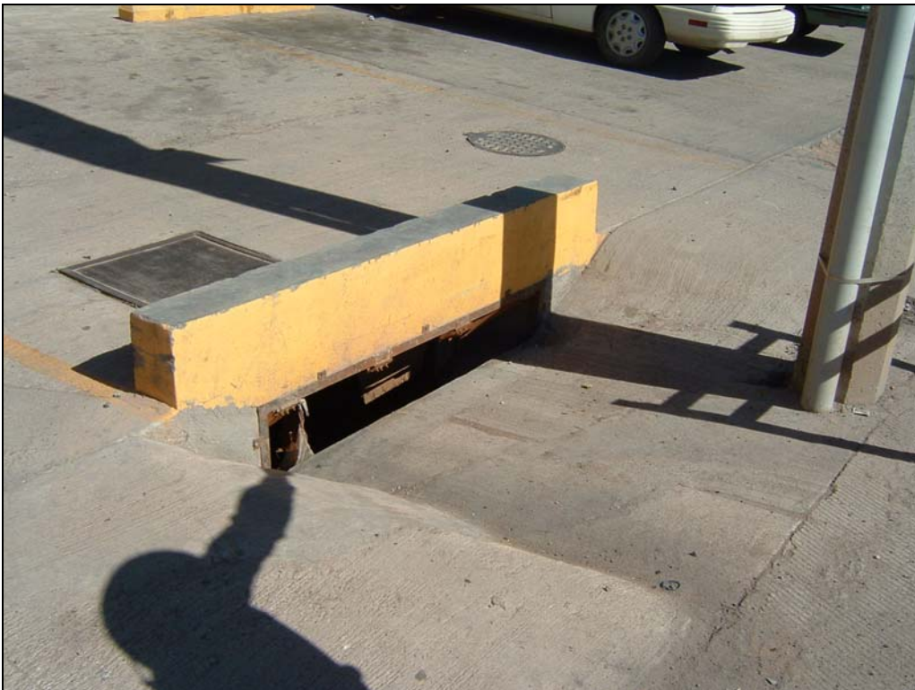
Figure 6. Undersized Tributary Inlet for Subarea L2 at International Highway.
