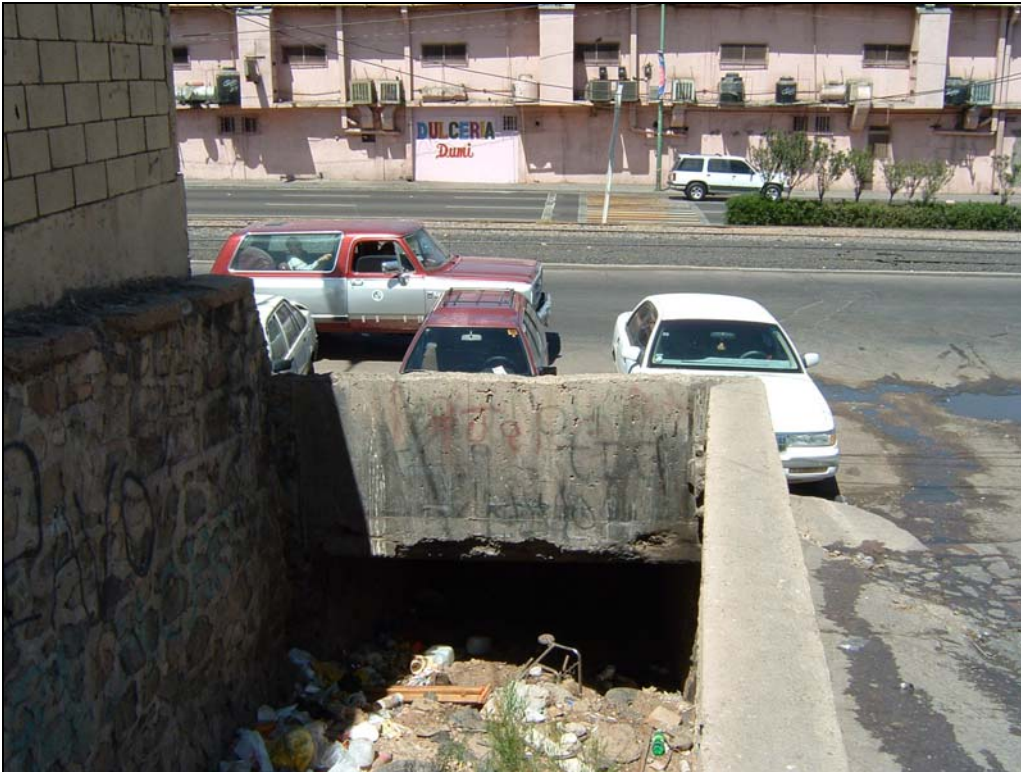
Figure 11. Tributary Inlet at Calle Embarcadero Alignment
