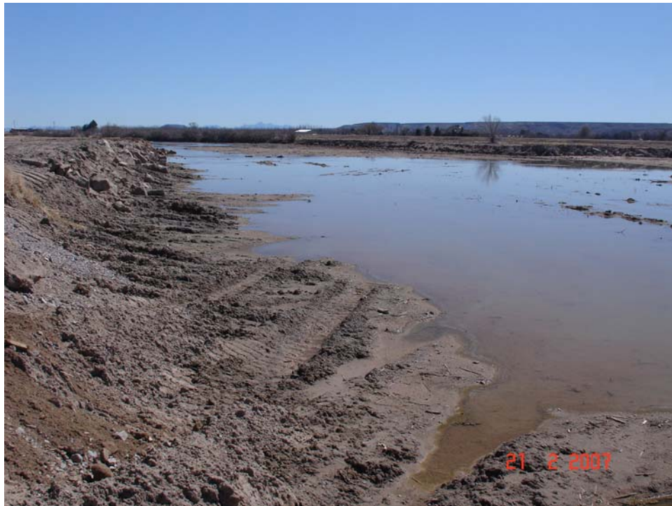
Figure A.48. View downstream of the excavated and reggraded channel of the Rio Grande at the mouth of Placitas Arroyo. The east bank has been reformed and armored with large rock and concrete rubble.
