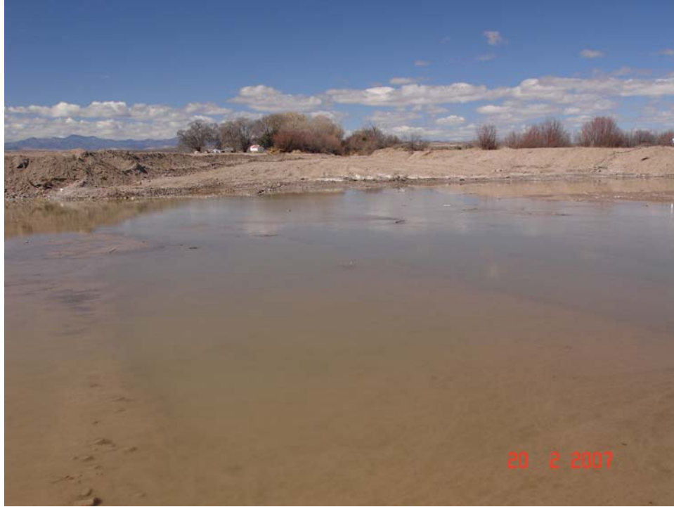
Figure A.39. View upstream of the reggraded lower reach of Trujillo Arroyo.
