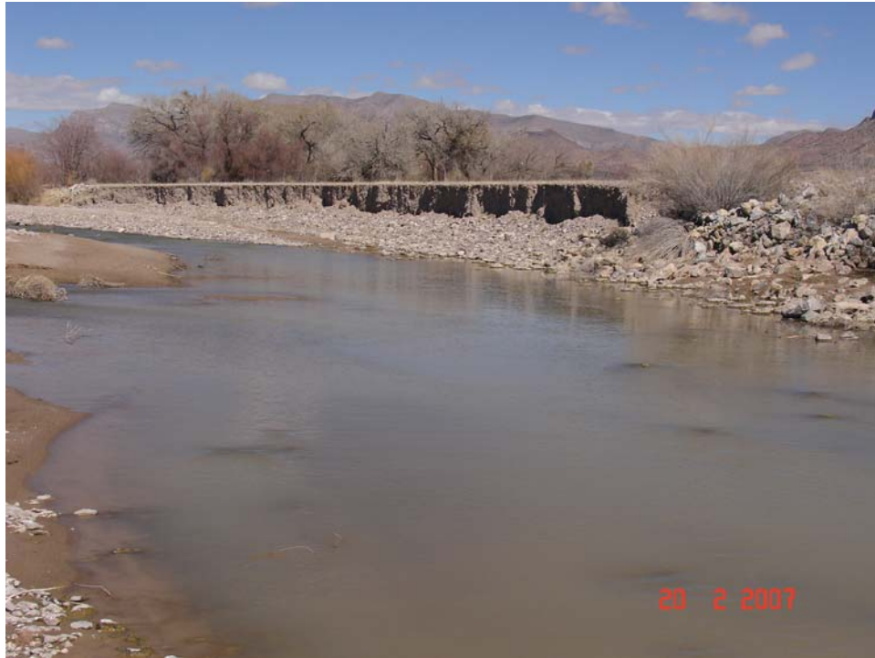
Figure A.5. View upstream of destroyed bank protection on the left bank of the Rio Grande at the confluence with Montoyas Arroyo.
