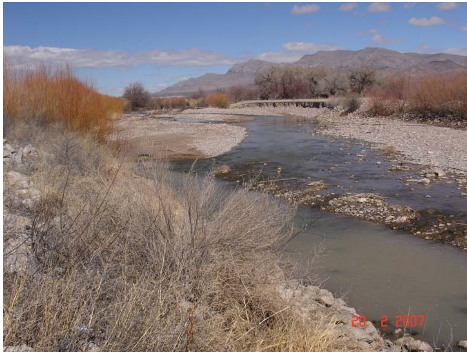
Figure A.40. View upstream of damaged bank protection on the east bank of the Rio Grande opposite the Montoya Arroyo debris fan.
