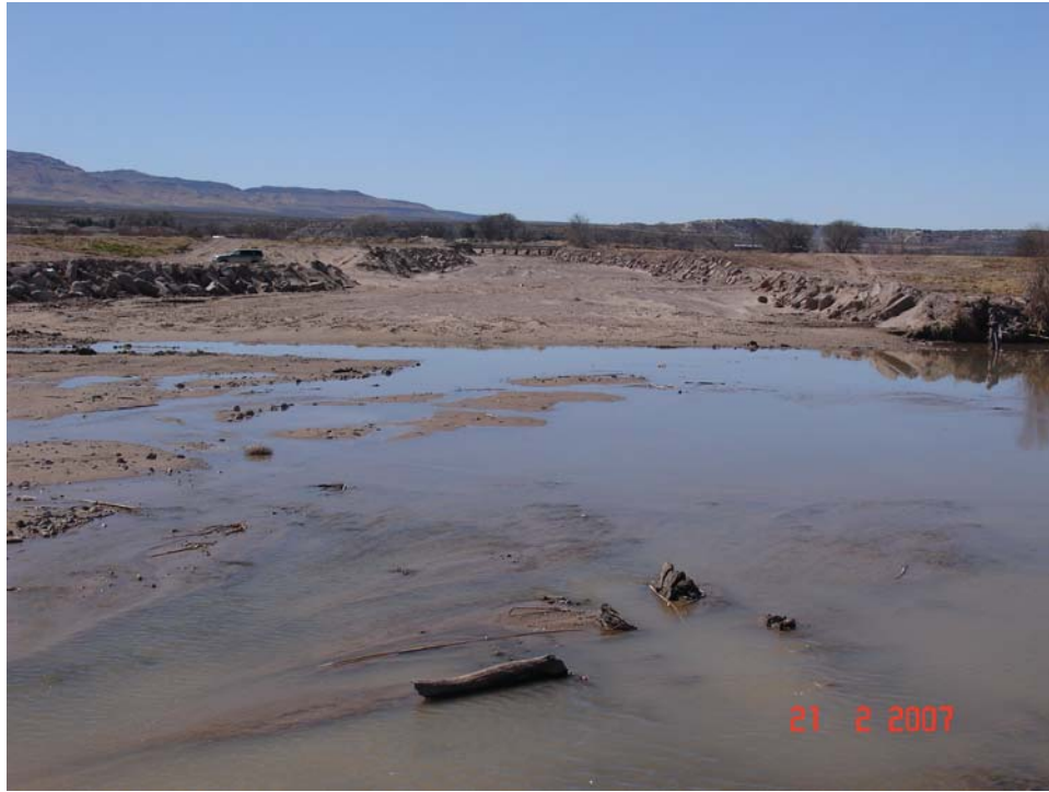
Figure A.47. View upstream of the excavated and reggraded channel at the mouth of Placitas Arroyo.
