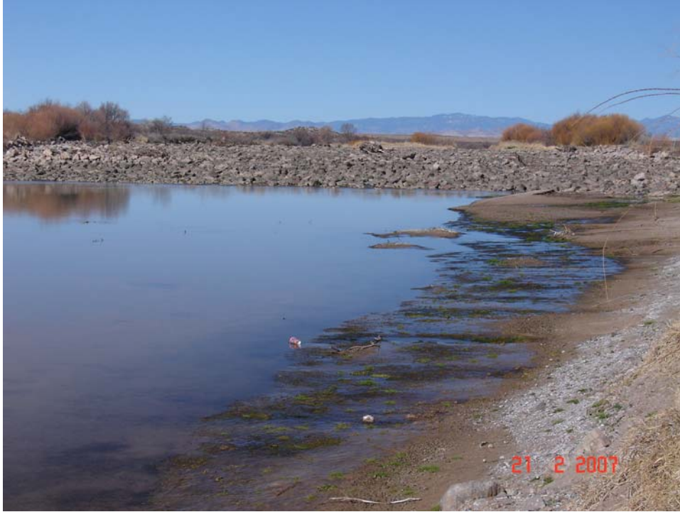
Figure A.35. View upstream of rock riprap protection at the Hatch Siphon at the downstream end of Subreach 1.
