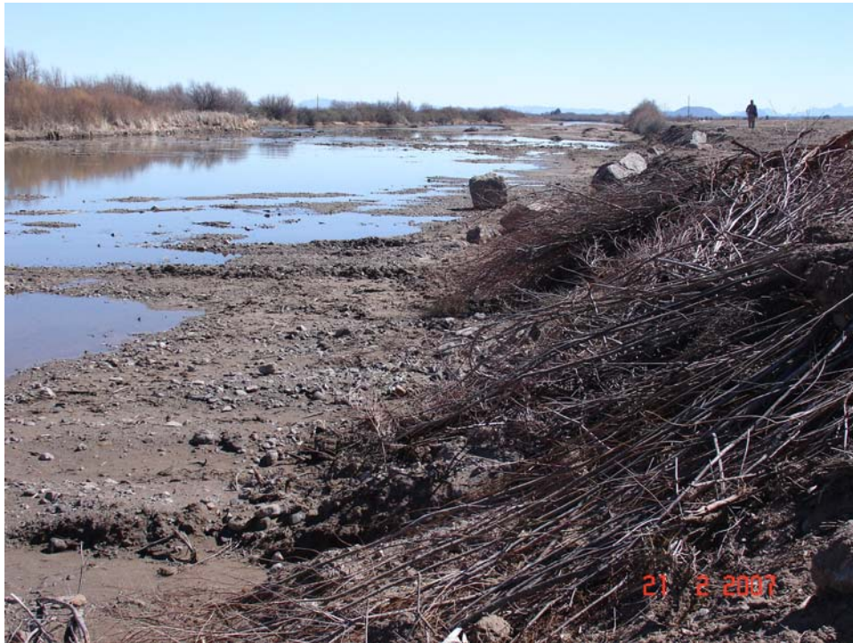
Figure A.9. View downstream of an excavated reach of the Rio Grande, and reconstruction and armoring of the west bank opposite Thurman I Arroyo in Subreach 2.
