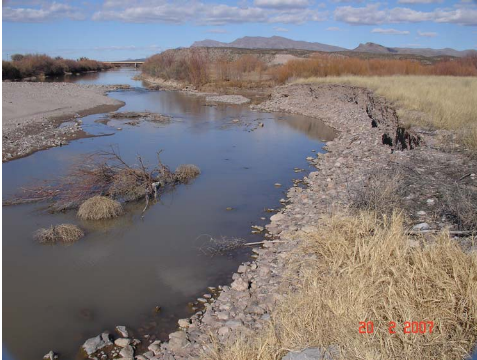
Figure A.41. View upstream of damaged bank protection on the east bank of the Rio Grande opposite the Tierra Blanca Arroyo debris fan.
