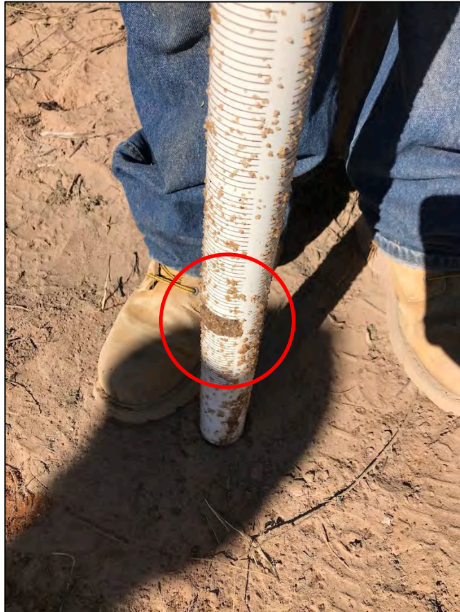
Figure 3. BW-MW-1 Original Well Screen
