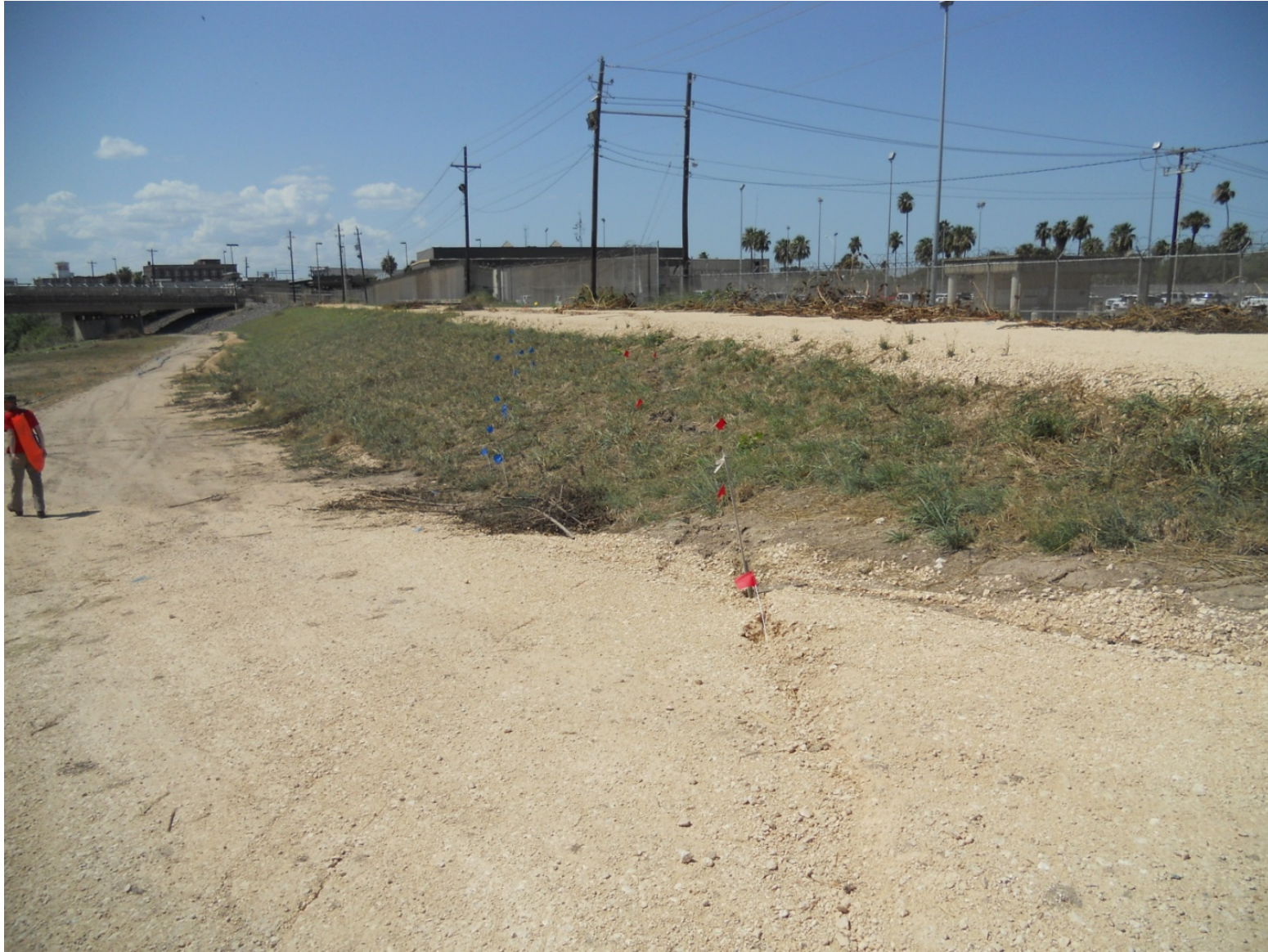
Figure 4.2. Two prominent cracks through the levee embankment at downstream end of study area that merge with cracks at the levee crest (see also Figures 1.2 to 1.4).
