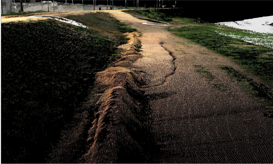
Figure 4.22. LiDAR image looking downstream showing the large crack separation at the toe, the crack crossing the gravel mound, and continuing upstream toward the viewer. White circular features in the image are the LiDAR stations where the instrument was placed to conduct the scan of the bank.
