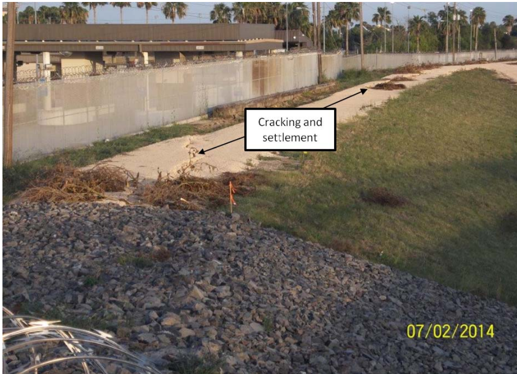
Figure 1.2. Severe cracking at the levee crest.
