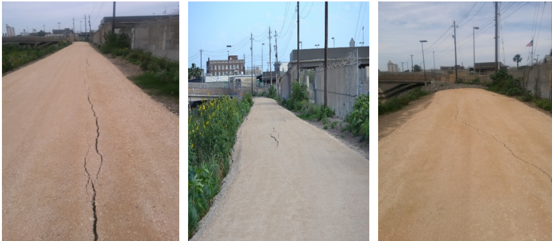
Figure 5.14. Photographs of levee cracking on 6 May 2014.
