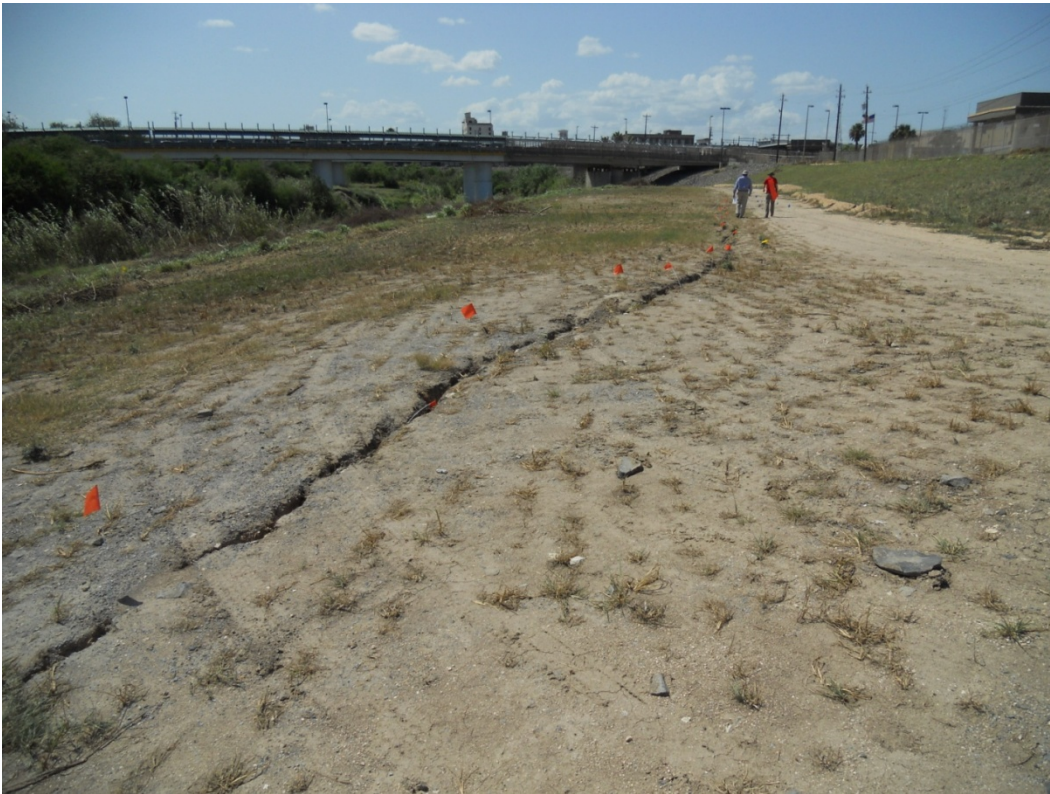
Figure 4.4. Longitudinal crack along the downstream end of the riverbank (see Figure 4.1 for location).
