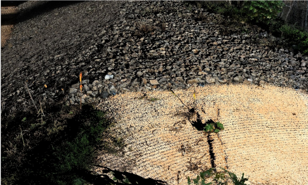
Figure 4.23. LiDAR image of the crack at the levee crest. Rip-rap at the upstream end of study area prevents examination of the ground surface to verify the upstream crack extent. LiDAR data does not provide additional resolution because of the coarse nature of the stone.
