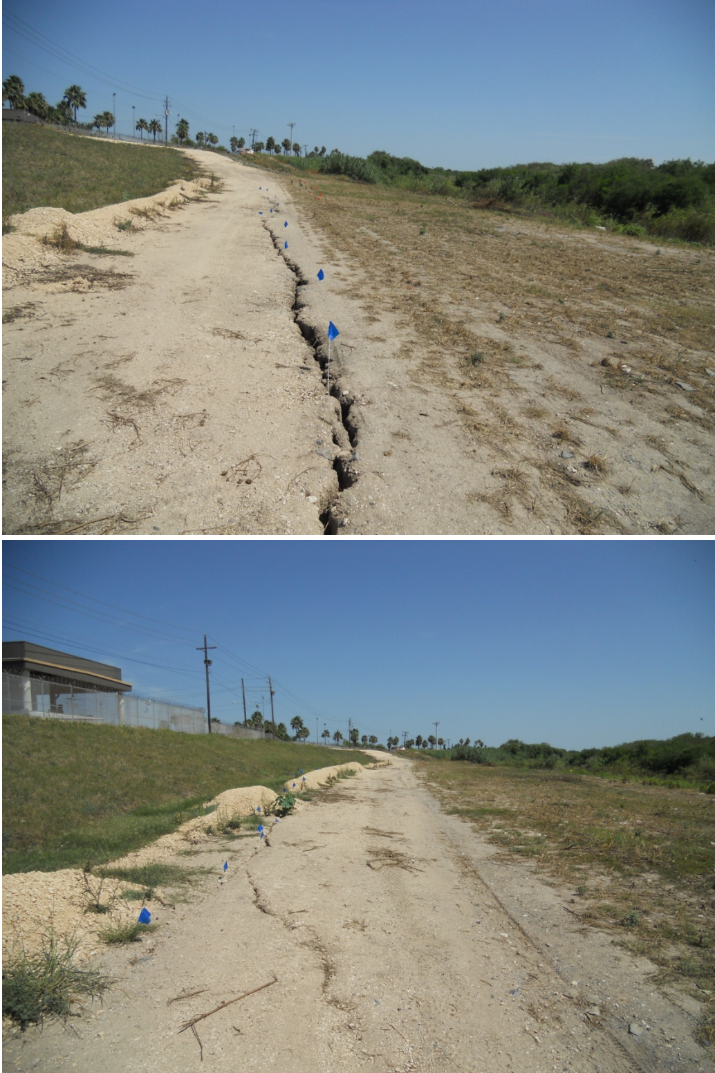
Figure 4.3. View of crack set at levee toe looking downstream. Crack extends through the gravel ridge in middle part of the lower photo and to the levee access road in top photo (see Figure 4.1 for location of crack).
