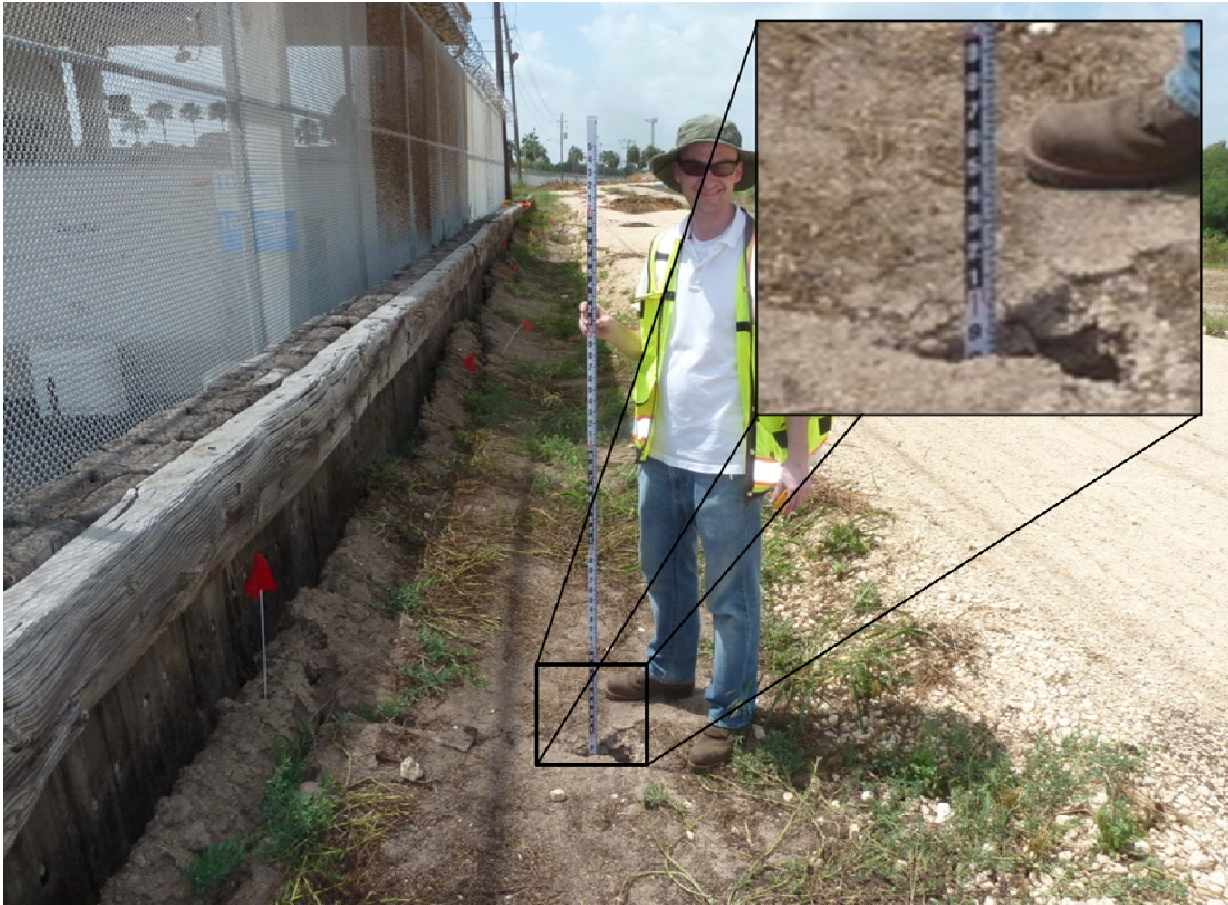
Figure 6.20. Depth of levee cracking, July 2014.
