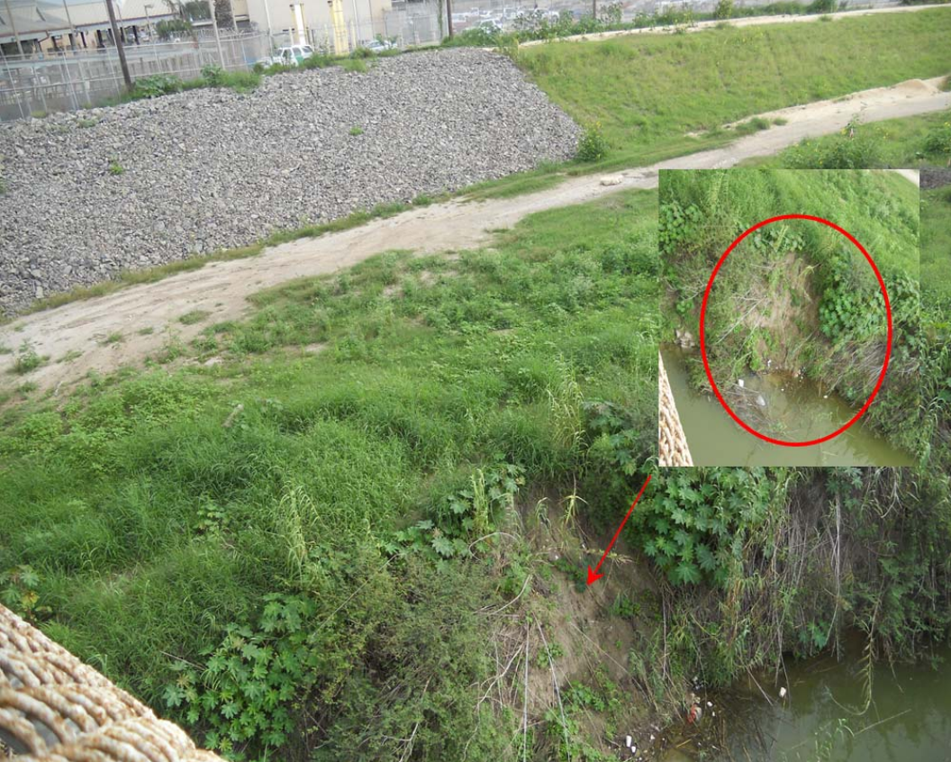
Figure 6.19. Minor riverbank sloughing in December 2014.
