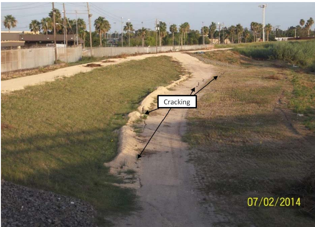
Figure 1.3. Severe cracking and settlement at the levee crest and at the waterside toe.
