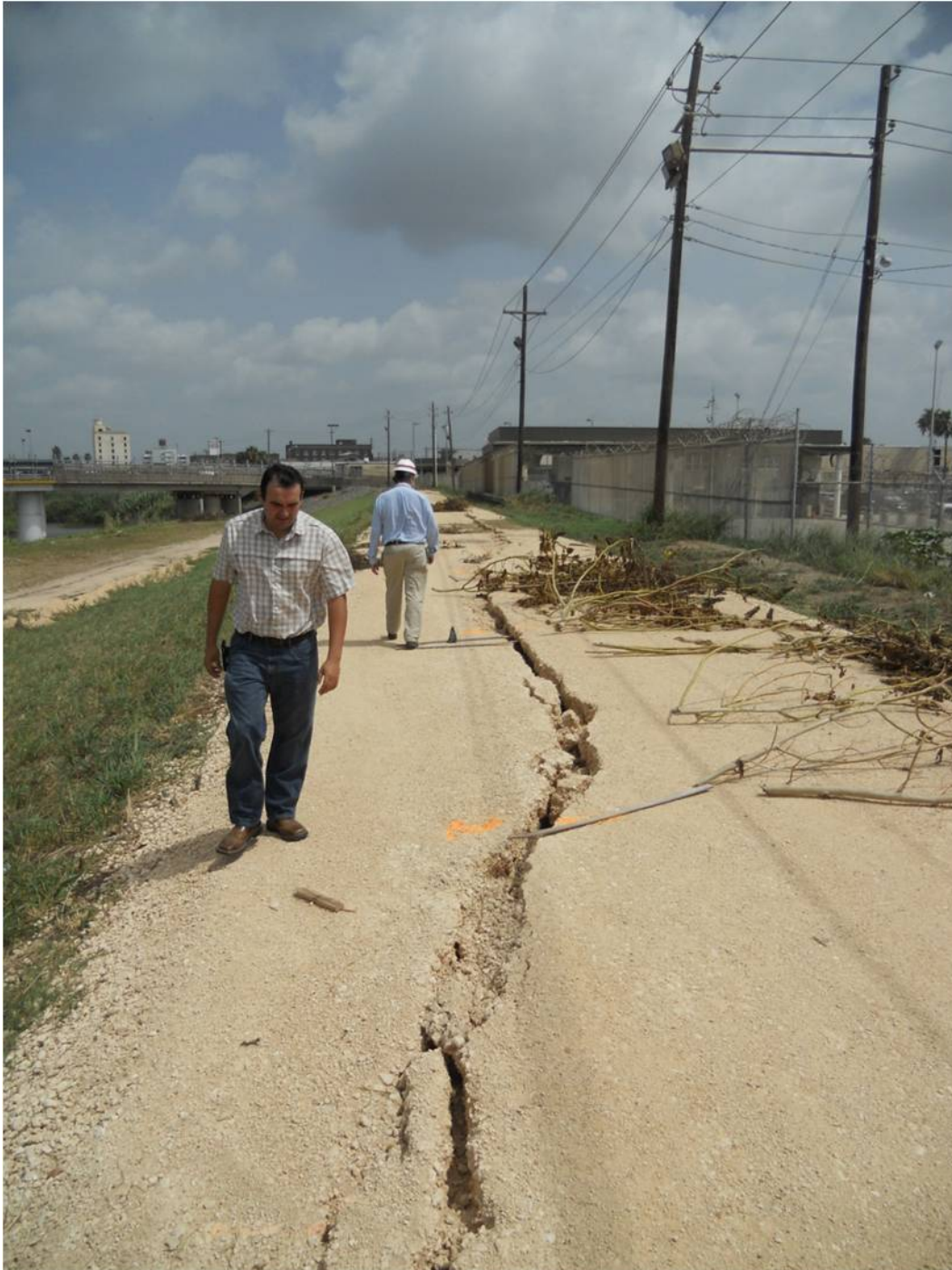
Figure 1.4. Close-up view of levee cracking and settlement at the crest. View is looking upstream. Gateway Bridge is in the background and corresponds to the upper limits of the study area.
