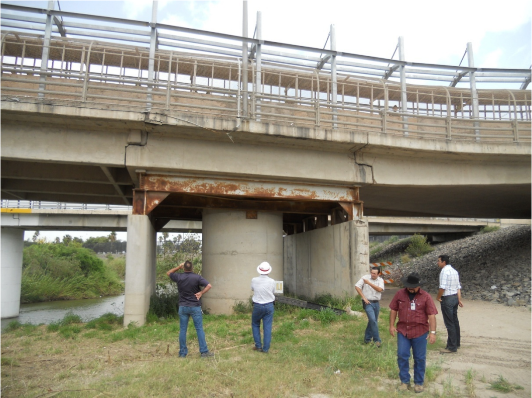
Figure 2.4. Support frame to remediate settlement of the International Gateway Bridge pier in 1984.
