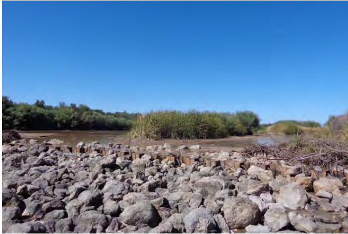
Figure 4-3. Hatch Siphon. Debris on Hatch Siphon sheet piling and island buildup upstream of Hatch Siphon, looking upstream, September 2013.
