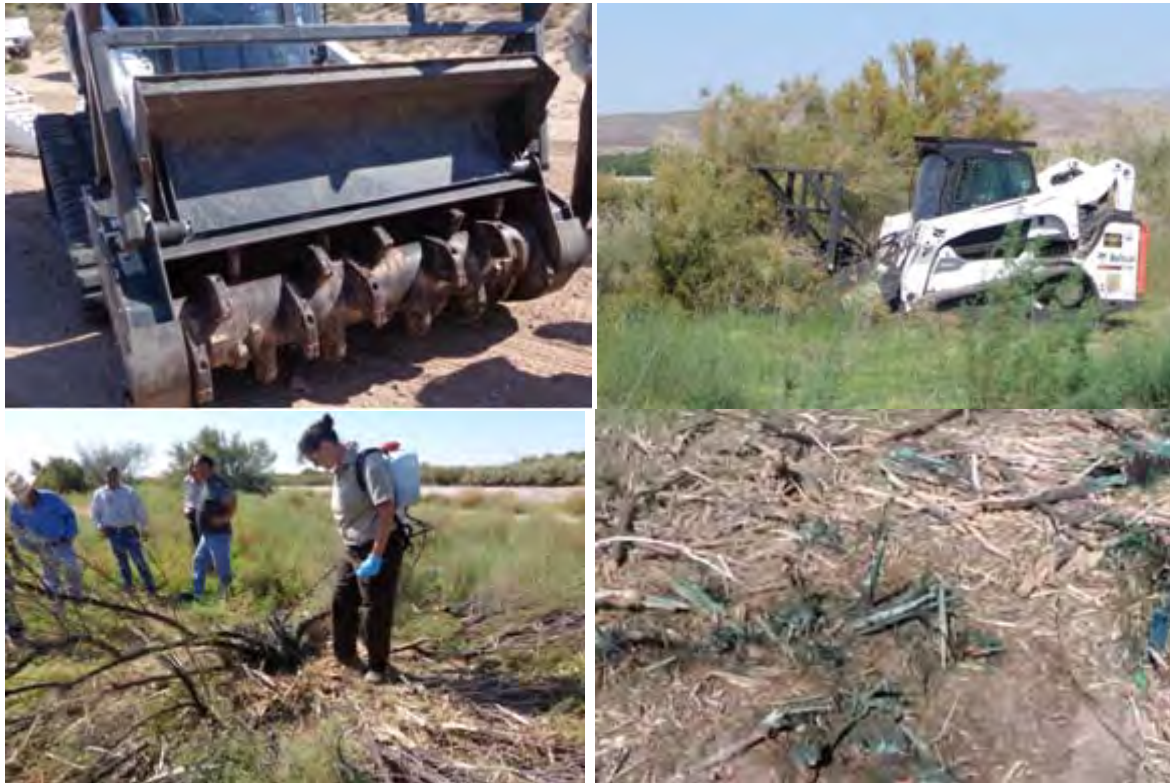
Figure 2-7. Mechanical and Herbicide Treatment method. A) Top left - example attachment on skid steer loader. B) Top right - equipment mulching large saltcedar. C) Bottom left - herbicide application on cut saltcedar stems. D) Bottom right - after herbicide.
