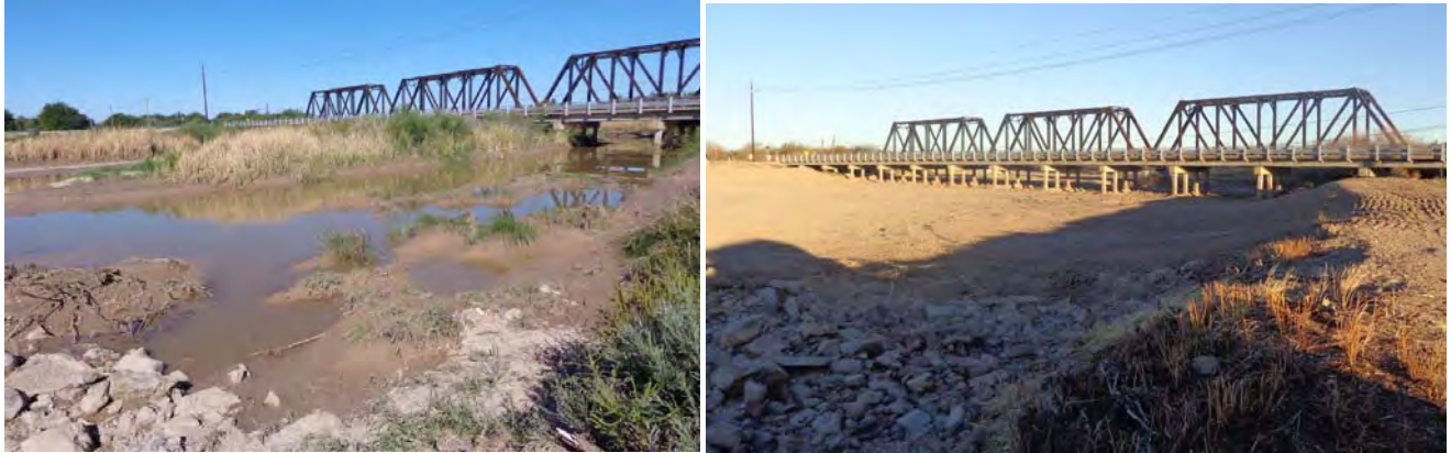
Figure 4-4. Looking upstream from Rincon Siphon, east bank. Left – Sediment accumulation and island formation upstream of Rincon Siphon, September 2013. Right – After excavation, March 2014.
