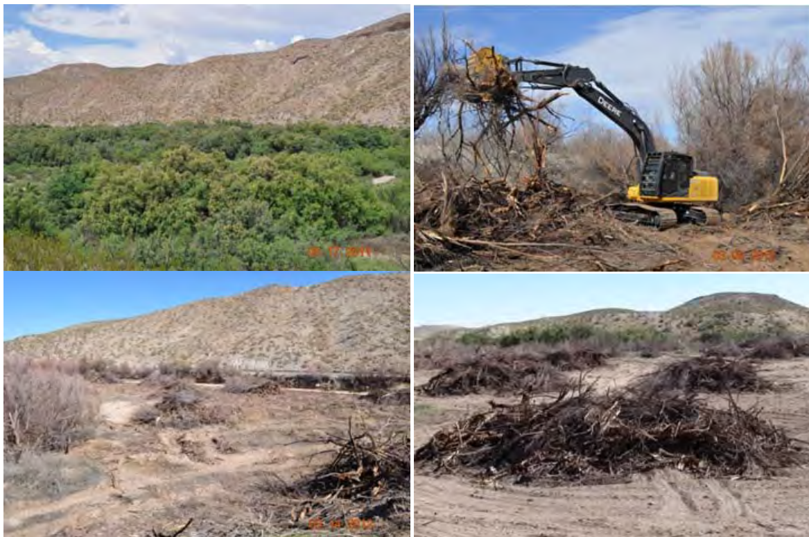
Figure 2-9. Mechanical Excavation Treatment method at the Broad Canyon Arroyo restoration site. A) Top left - example of monotypic stand of saltcedar. B) Top right - equipment excavating saltcedar. C) Bottom left - landscape after excavation. D) Bottom right - debris piles.
