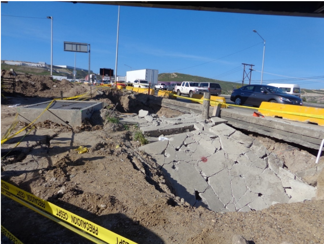
Figure 10 Additional damage along roadway due to collector collapse downstream of junction box- Blvd Lazaro Cardenas, Colonia Los Pirules, Tijuana, B.C. - March 9, 2017
