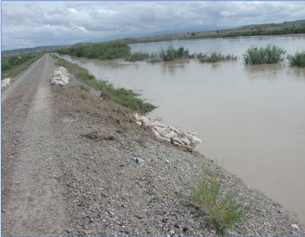
Presidio levee during 2008 flood
