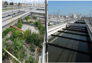
Before and after: Sediment and debris accumulation in a primary sedimentation tank resulting in reduced capacity and compliance issues.
