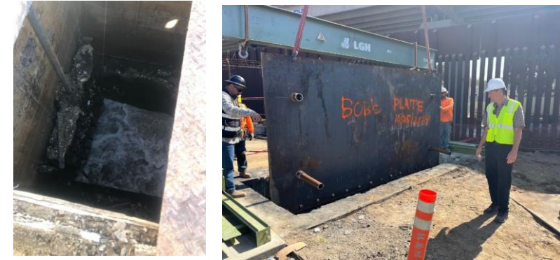
Joint Box Valve 96 inches not functioning
