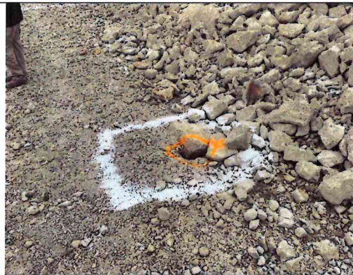
February 21, 2024 Sinkhole #53 is identified at the toe of the upstream slope at Station km 5+560.
