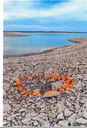
February 26, 2024 Sinkhole #54 located at Station km 5+450 was observed 320 m away from the toe of the upstream slope.
