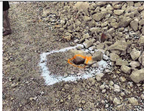
February 21, 2024 Sinkhole #53 is identified at the toe of the upstream slope at Station km 5+560.
